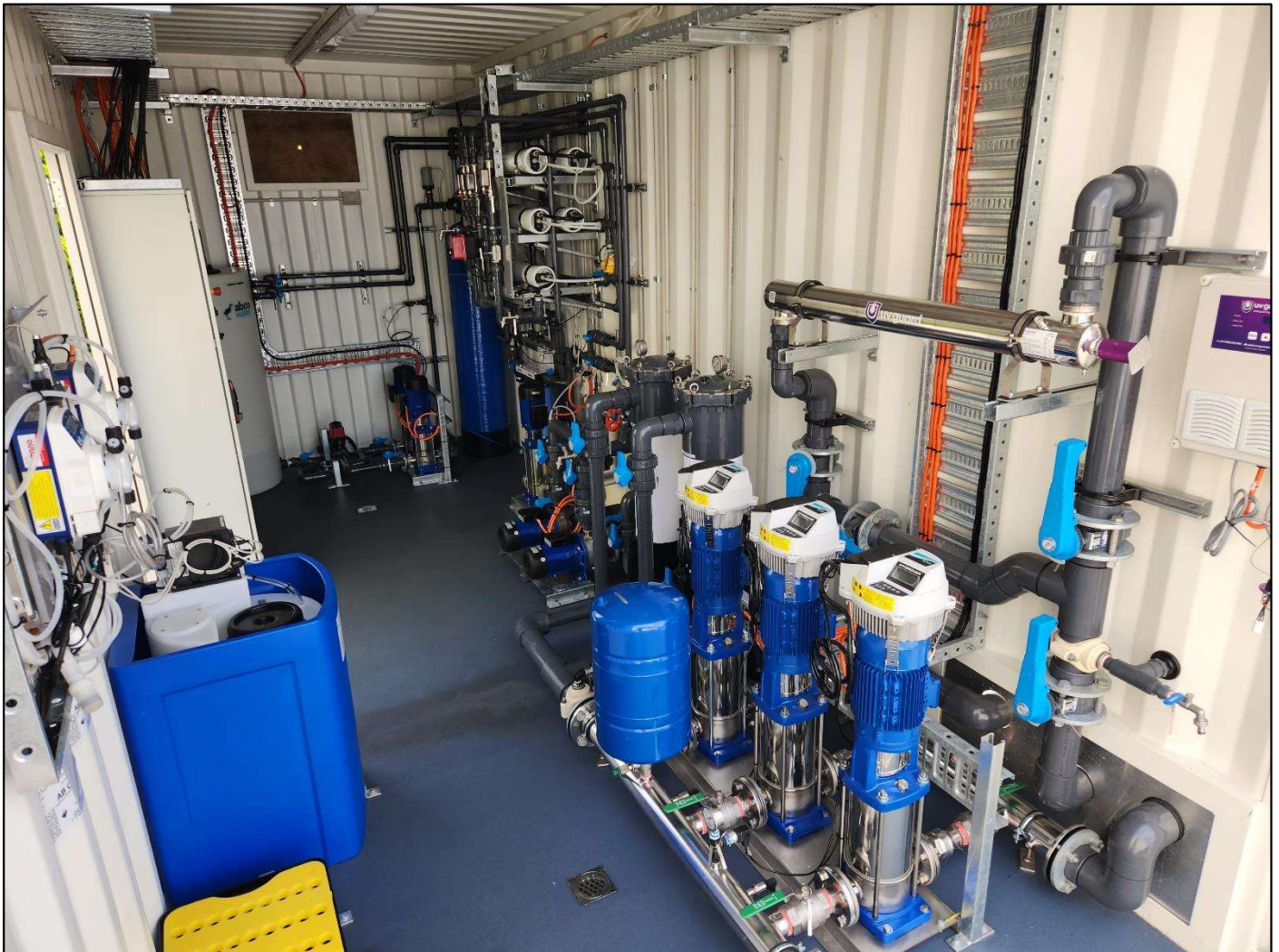
ABCO 24 m 3 /day containerised RO plant
