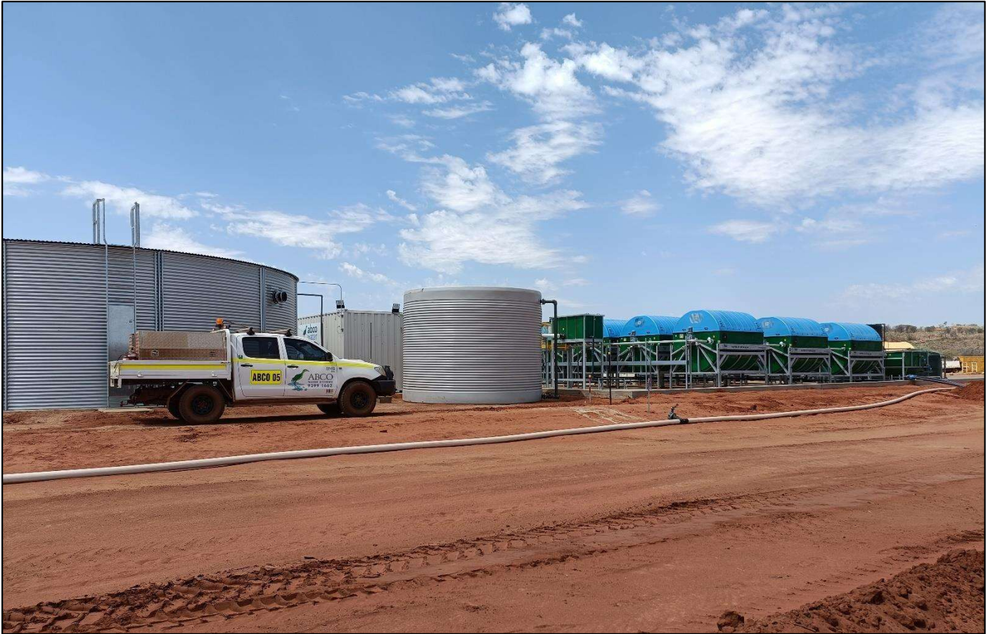
ABCO PWTP and WWTP installed onsite
