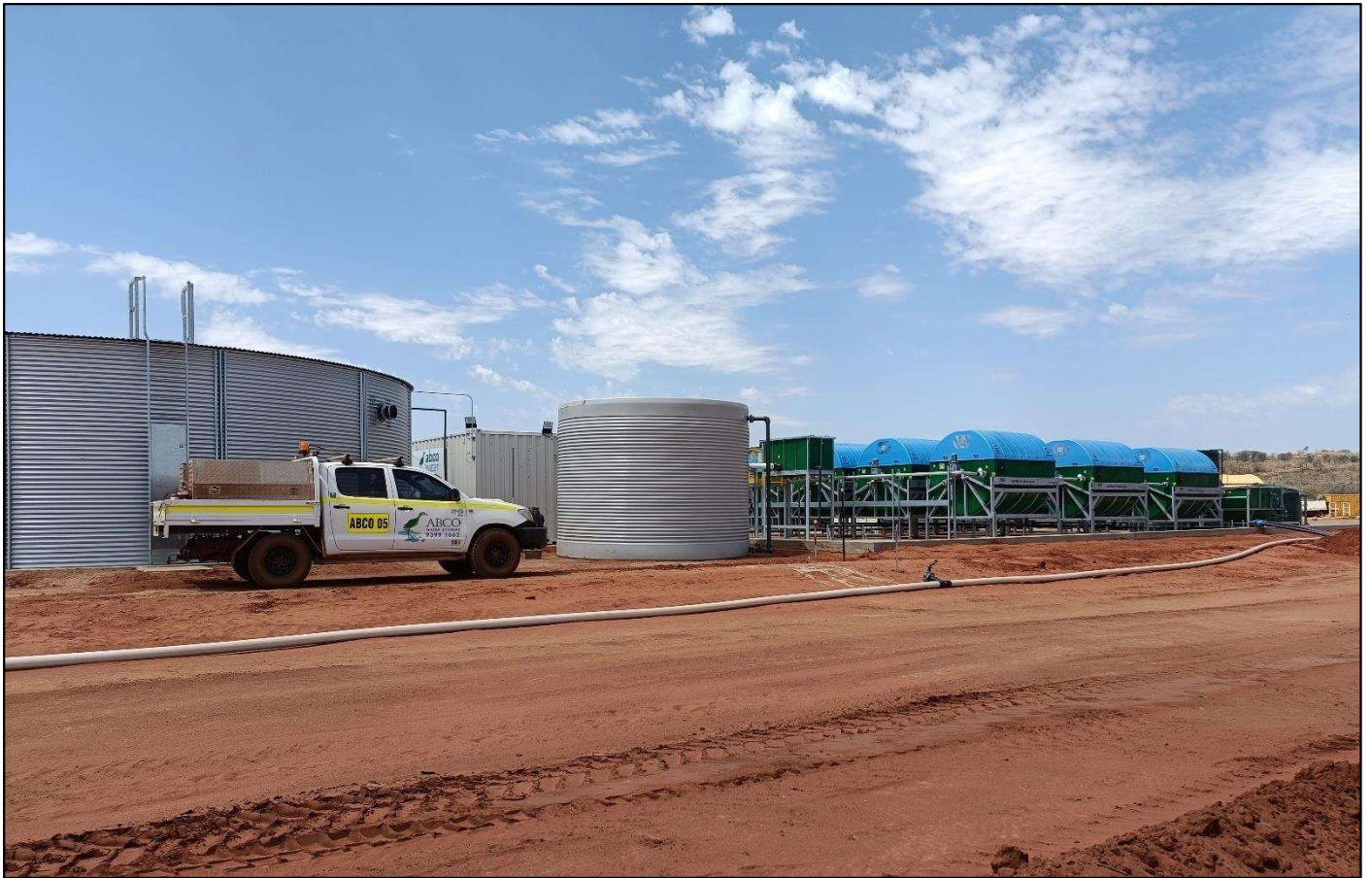
ABCO PWTP and WWTP installed onsite
