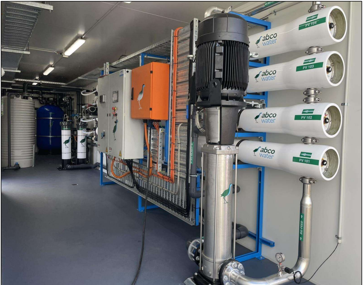
ABCO 480 m 3 /day containerised RO plant
