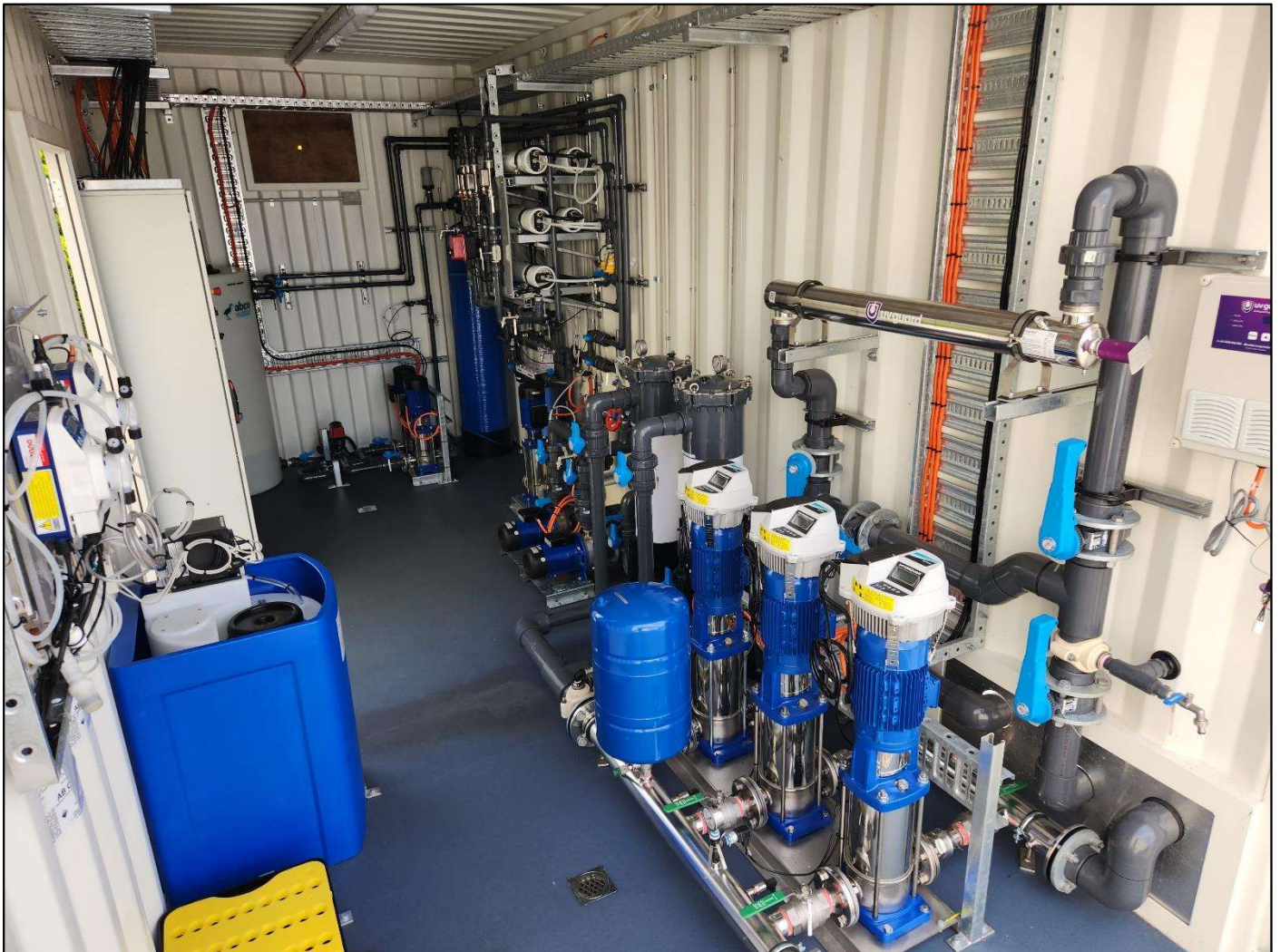
ABCO 24 m 3 /day containerised RO plant
